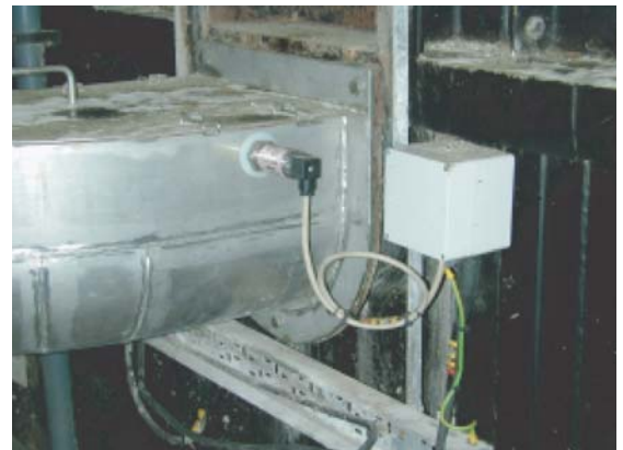
Figure 2: The Compact Vibrating Fork Level Switch installed in the horizontal half cylinder wash water channels.
