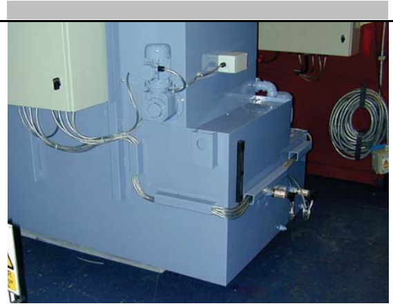
Figure 3: Two Compact Vibrating Fork Level Switches used in a larger filtration unit.
