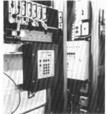
One switch of the automatic dialing remote monitoring systems, which are located on the front panel, controls the release of alarm data from the PLC to the dialer, switches the phone line wires into the dialer, and places the system in the desired operating mode.
