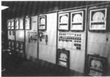
Wolf Creek Highway Water District's SCADA system head-quarters facility consists of six 42-in. bays containing conventional operator interface devices such as recorders, switches, meters, and alarm indicators. Microprocessor controlled PLC subsystems, automatic dialing remote monitoring systems, and dedicated communications modules are located behind the panels.
